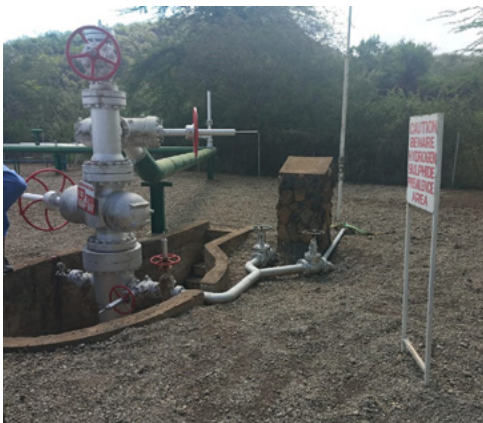
Geothermal well used for green house heating at Oserian Development Limited
