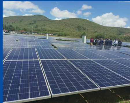
1MW Solar Photovoltaic Plant used for operations at Oserian Development Limited
