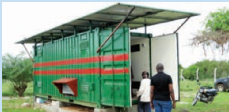
Solar milk cooling station installed by Techwin Limited at Garsen cooling plant – Tana River County
